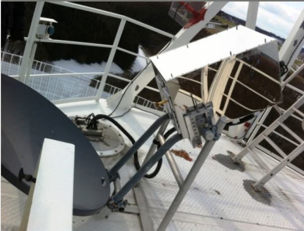
Figure 1: The WVR is installed permanently on the Effelsberg on focus cabin roof and is oriented boresight to the observing beam. The radiometer beam is conical with FWHM of 2.6° matched to the cylindrical Effelsberg main beam for maximal beam overlap in the first 1 km of atmosphere where most of the water vapour typically lies.
